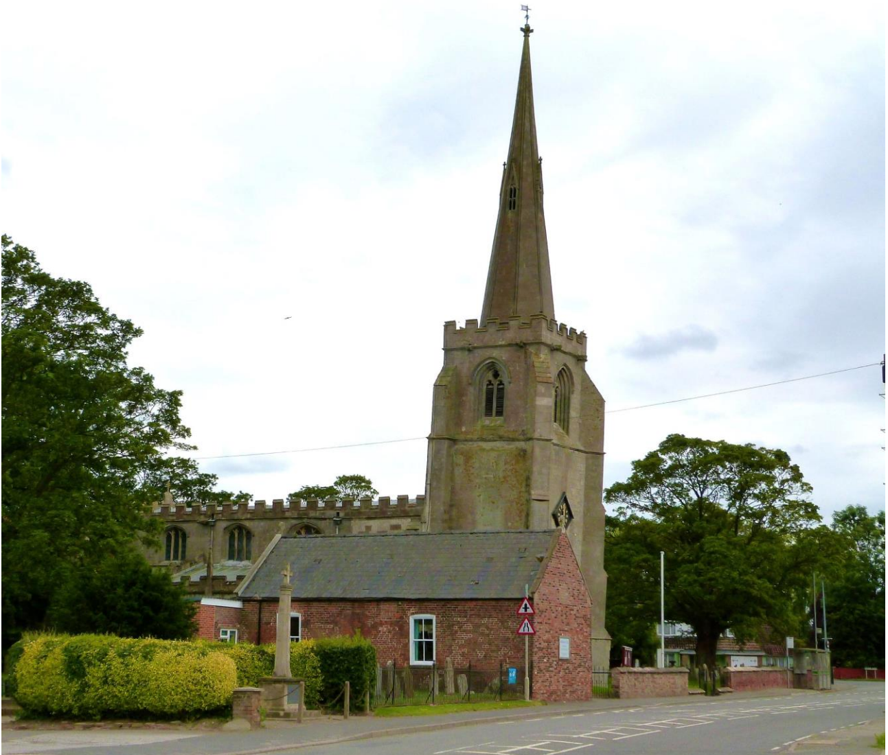
Figure 11 The tower and spire of St Lawrence church at Surfleet which shows evidence of subsidence.
