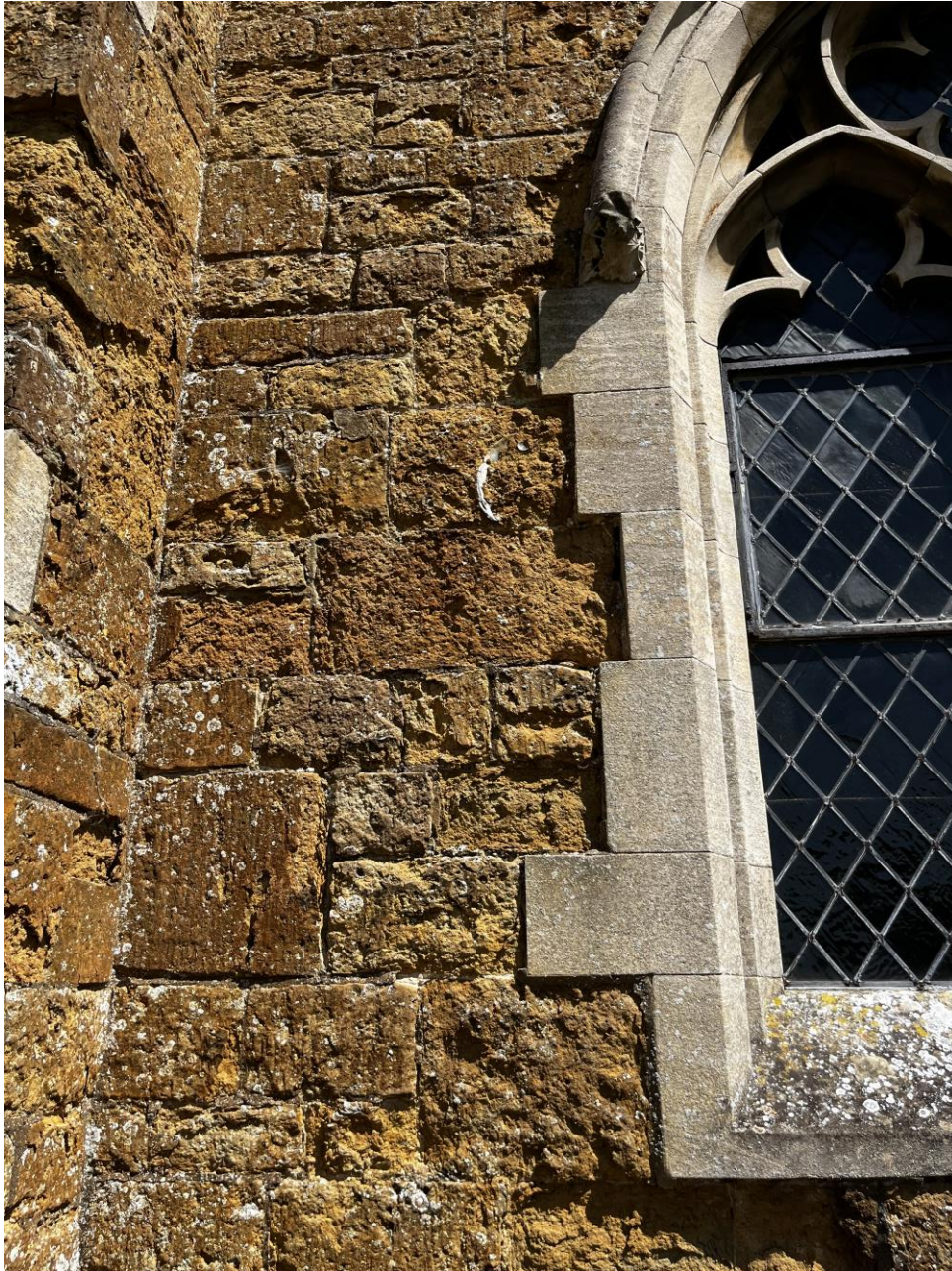
Figure 30 Ashlar of Tealby Limestone in the church at Nettleton. Note the large bivalve ( Camptonectes cinctus ) visible in one of the blocks. The quoin stones are of Lincolnshire Limestone.
